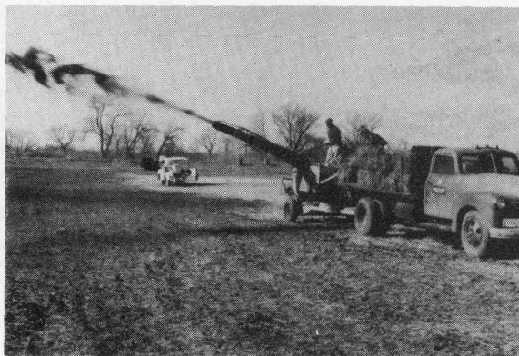
Figure 9.--Blower-type mulch spreader showing application of a mixture of hay and asphalt. This spreader can be used on short slopes such as highway right-of-ways. It can be equipped with extension pipes and hoses for use on longer slopes.
