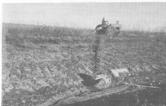
Figure 16.--Leveling small rills on 3:1 slope with slope harrow in preparation for seeding and mulching. The weight at the bottom prevents the harrow from pulling up the slope.
